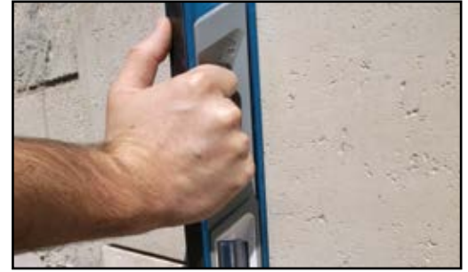
Use a large level to check and maintain an even-face plane over multiple tiles.
