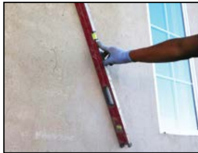
Use a long level or straight edge to confirm your wall is flat.
